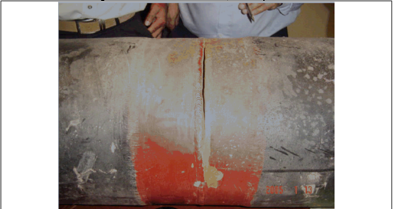
Figure 9. Photo of December 22, 2004 Pipe Break
